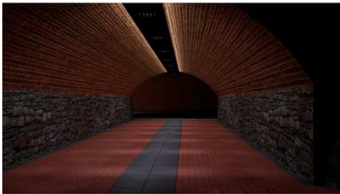
Paxton Tunnel lighting feature
